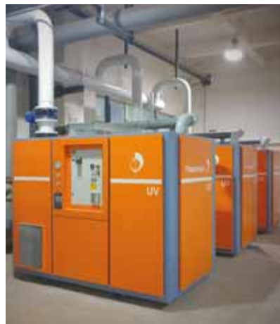
Pneumofore UV50 VS90 Vacuum Pumps at Changyu Glass - China
