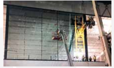
Installation of the oversized façade elements at the Tesla factory in Austin, Texas, USA - © W&W Glass
